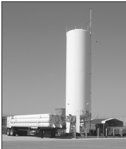
LINWELD's Liquid Hydrogen facility. Liquid Hydrogen is stored in cryogenic vessels at temperatures below -423° F.
