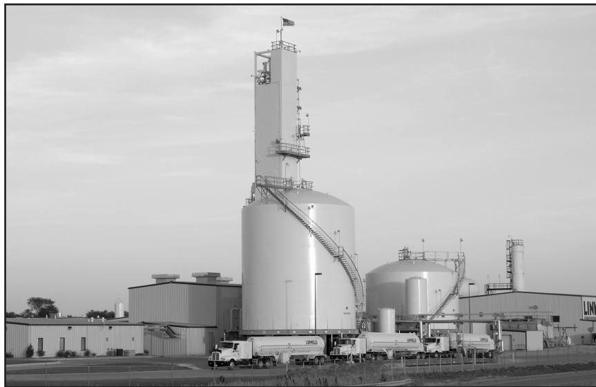
LINWELD's Coyote Air Separation Production Plant, located on the LINWELD Campus, Waverly, NE.
